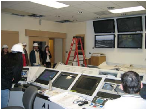
CENTRAL MANAGEMENT FACILITY
